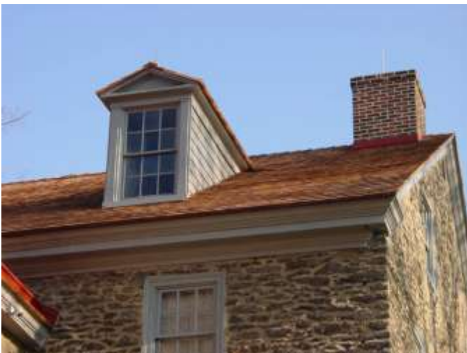
A view of the new roof of cedar shakes, one of the rebuilt chimneys and new gutters and flashing.
